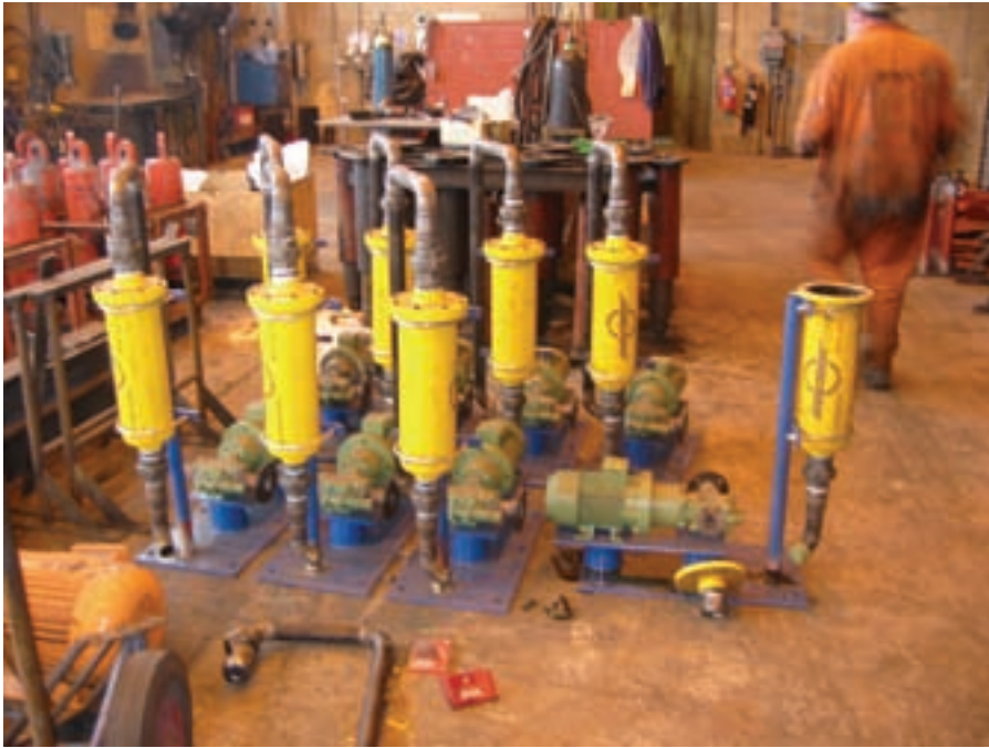
Figure 4 —Magnum installation at the Didcot A Power Station in England.
