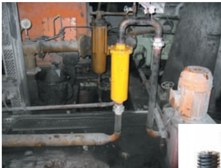
Figure 1—Magnum installation at Rugeley Power Station.
